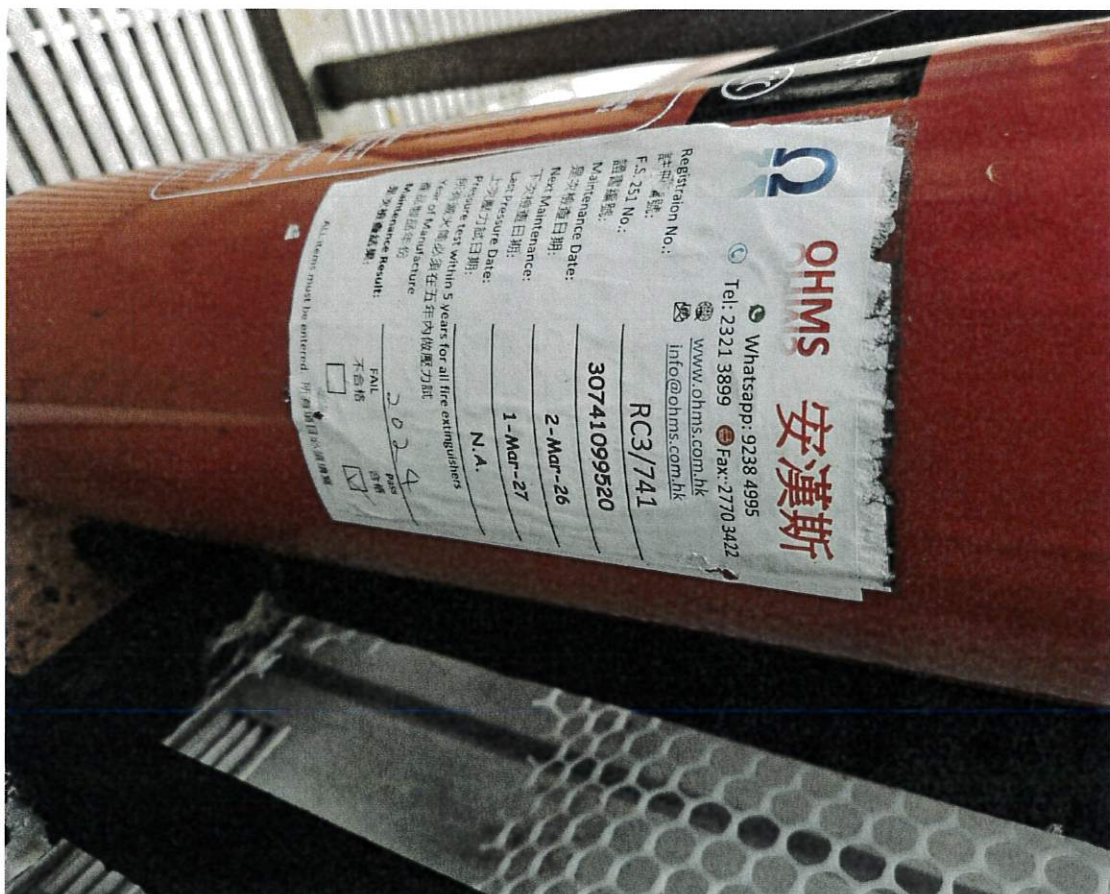
Installed Fire Extinguisher Information
